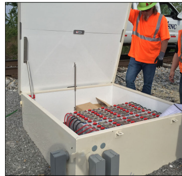
(20) SUN+660 Batteries & Battery Box
