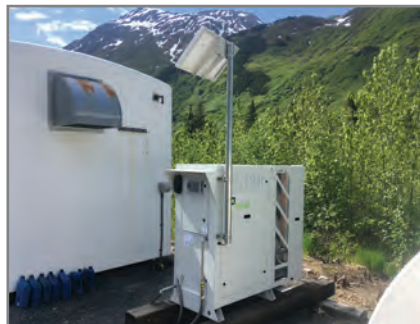
Test site with major railroad in Alaska. PowerGen is used to daily cycle charge a 48V battery bank at a remotely located telecom location along the wayside.
