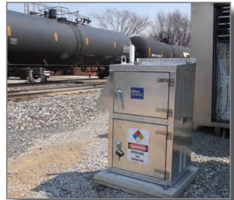
1st SOFC installed with major Class I railroad at busy grade crossing in North Baltimore, OH.
