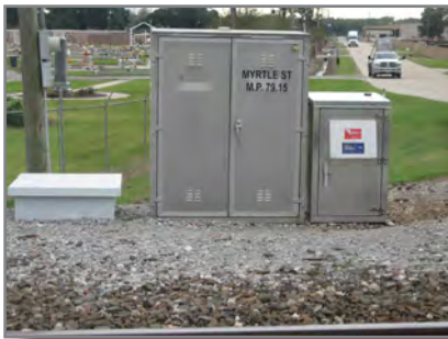
Project with major Class I railroad to "harden" mainline track along Gulf Coast
